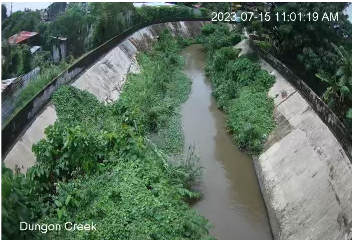
Narrow channel at Dungon Creek with paved creek banks reducing absorptive capacity of the land
